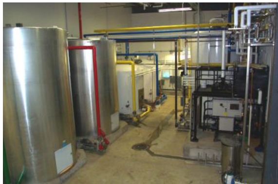
Batching / Tank Room & Controls
