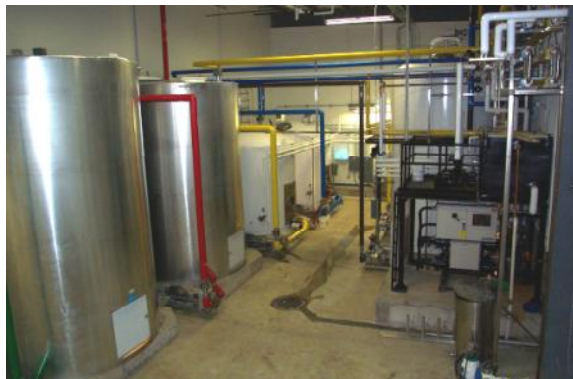
Batching / Tank Room & Controls
